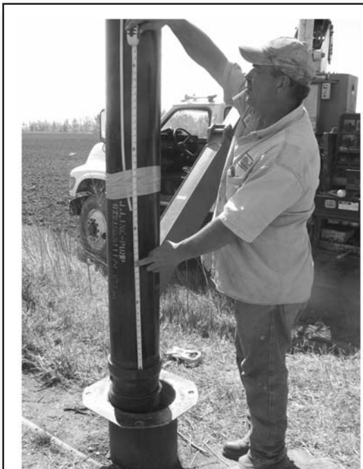
Figure 1. Irrigation Central staff out of Sikeston, MO tie in the bottom of the air line a few feet from the pump.
